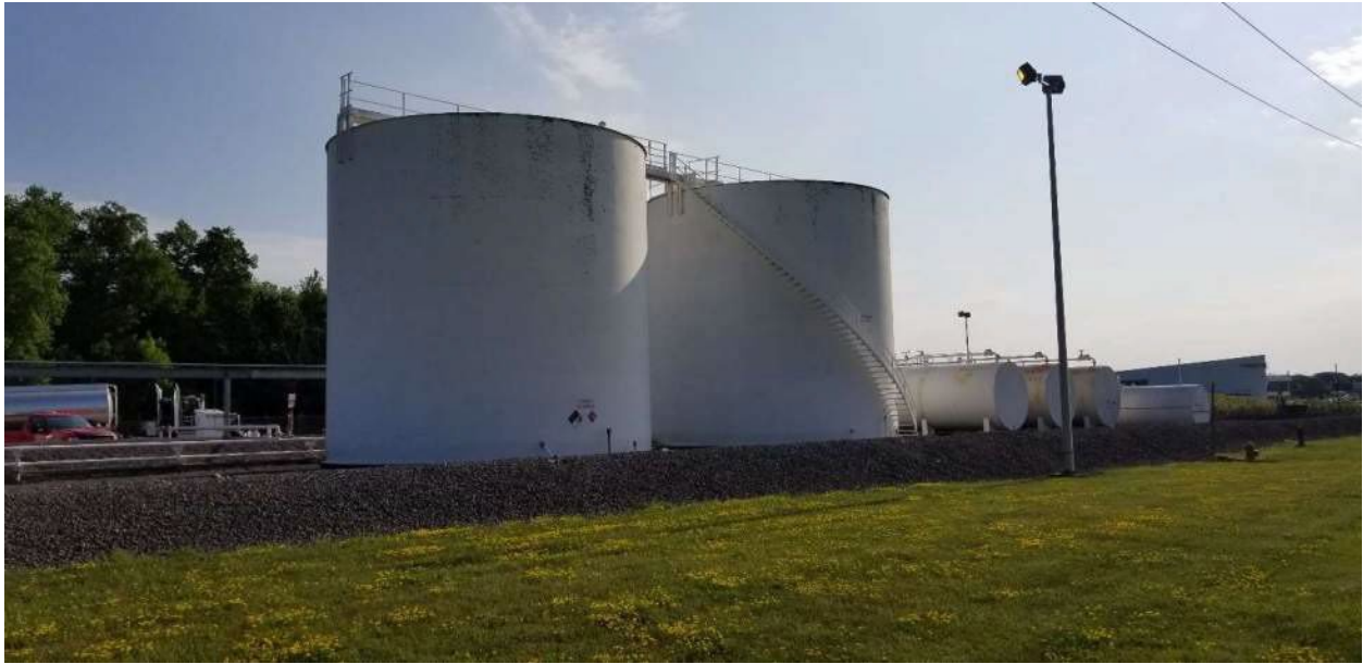
Figure 7 – Jet A Tanks
