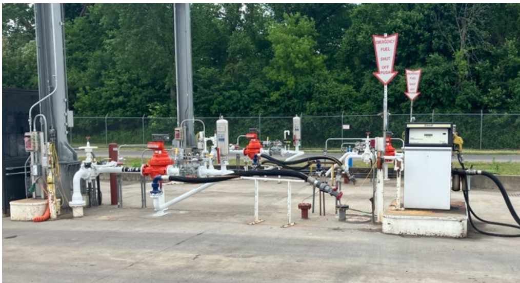
Figure 4 – Jet A Only Loading Island (No. 2)
