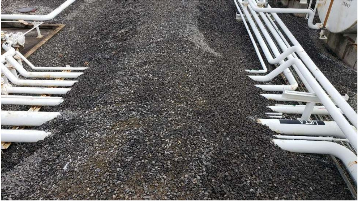
Figure 9 – Buried Product Piping
