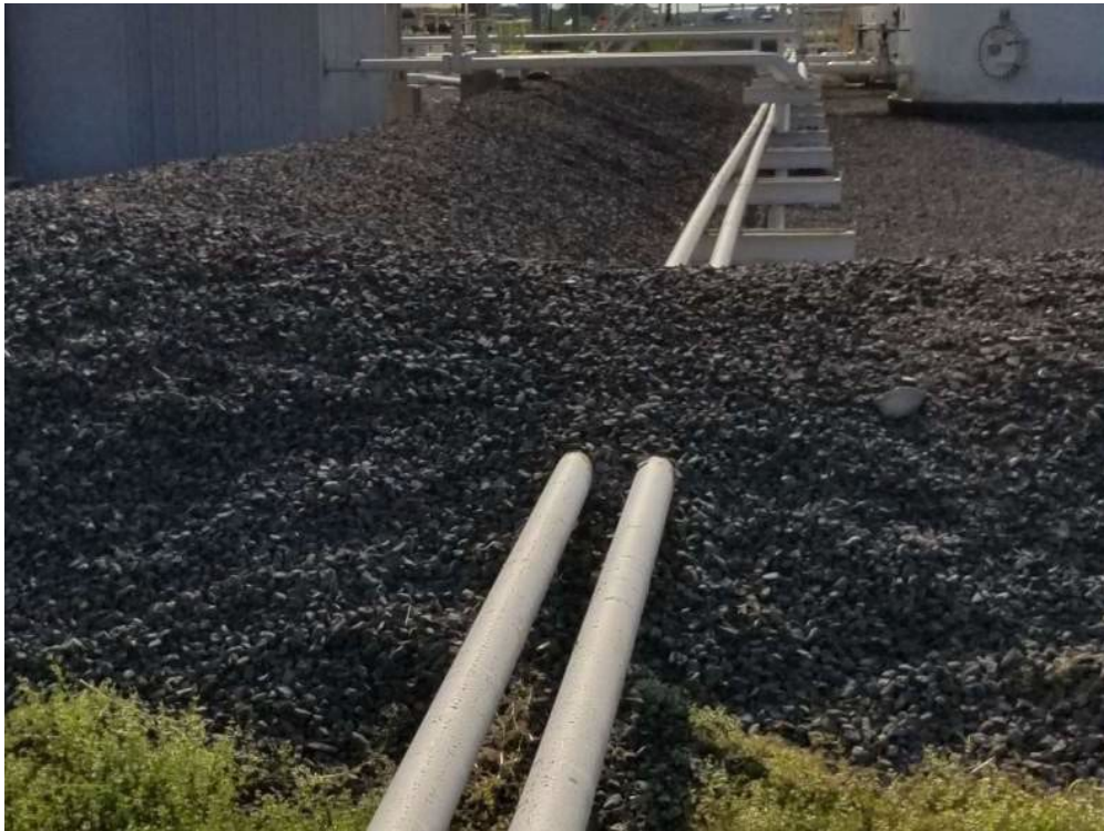
Figure 10 - Buried Product Piping
