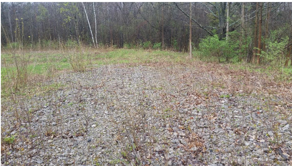
View of the crushed concrete and block remaining in the footprint of the previously demolished U.S. Air Force base housing complex.
