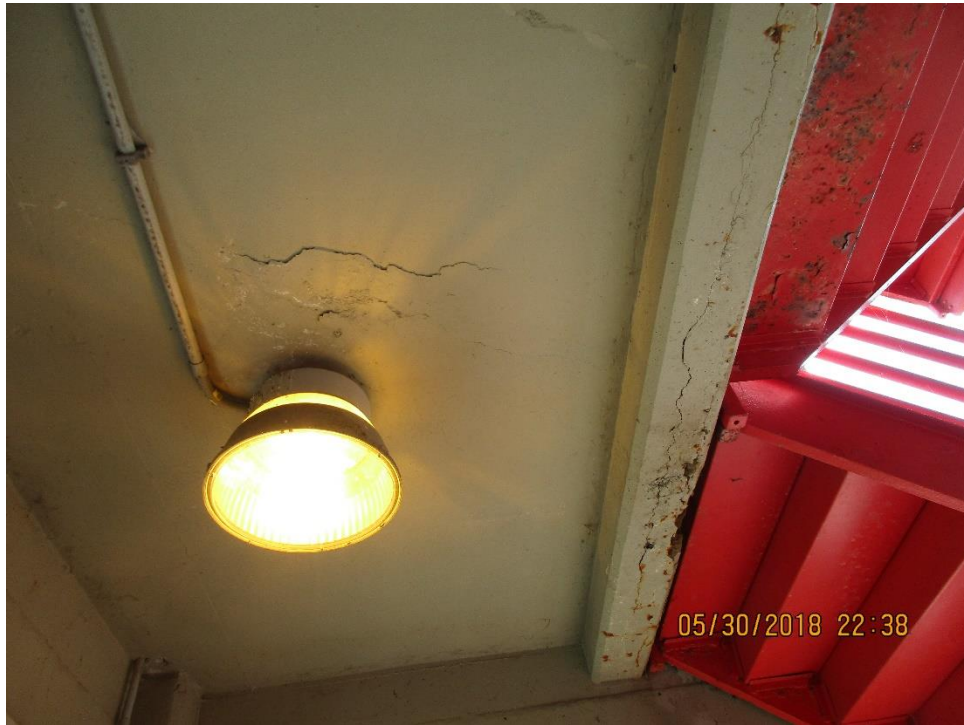
Photo #27: Stair tower #3 – cracked beam and soffit of Level 3 landing
