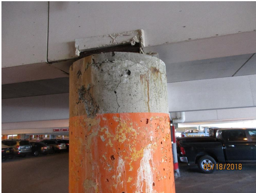
Photo #1: column S3 on Level 3 - hairline cracks at top of column
