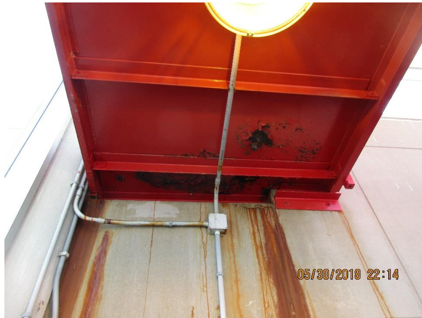
Photo #25: Stair tower 4 – Corrosion of steel pan of landing and water stains running down side of wall
