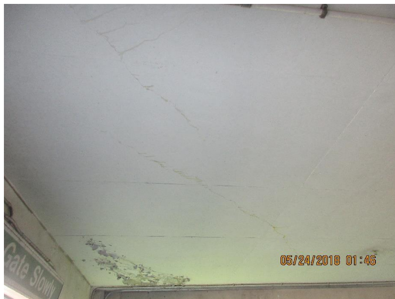
Photo #14: Hairline cracks at Northeast corner Level 2 soffit
