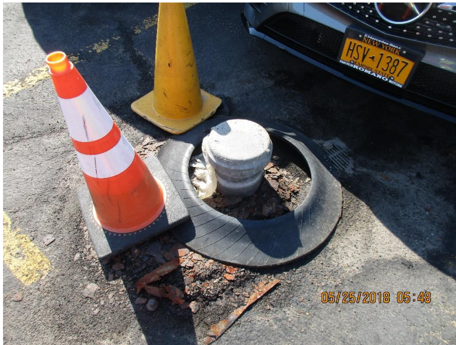
Photo #23: missing steel bollard around utility.
