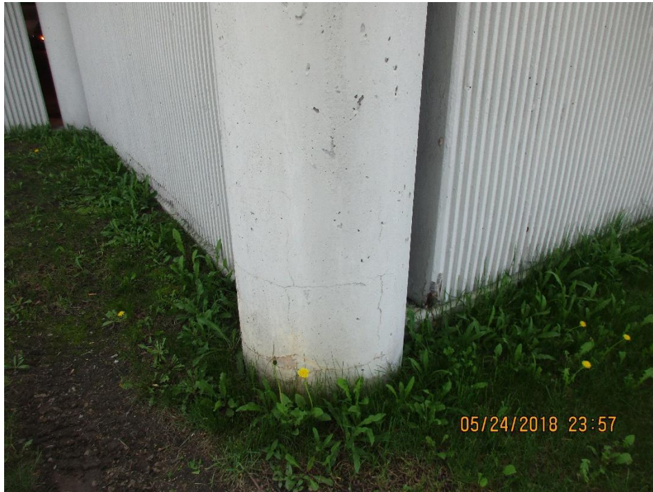
Photo #9: typical concrete column cracking at base.
