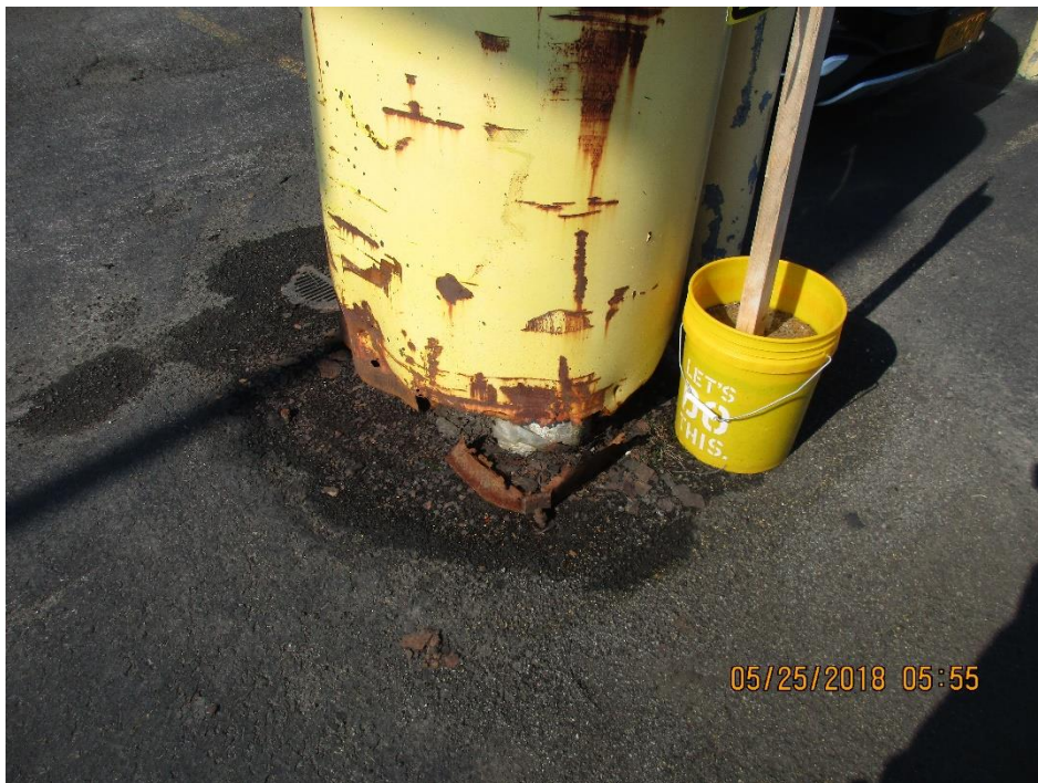
Phot #24: Damaged and displaced steel bollard.
