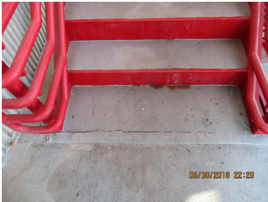
Photo #26: Stair tower 3 – cracked stair pan
