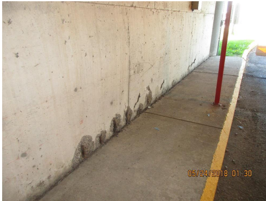
Photo #13: North West garage entrance ground level spalling and corroded reinforcing on wall
