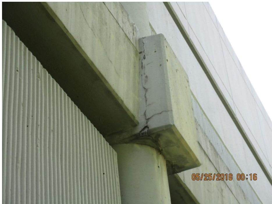
Photo #16: Cracked post tensioning pocket cover
