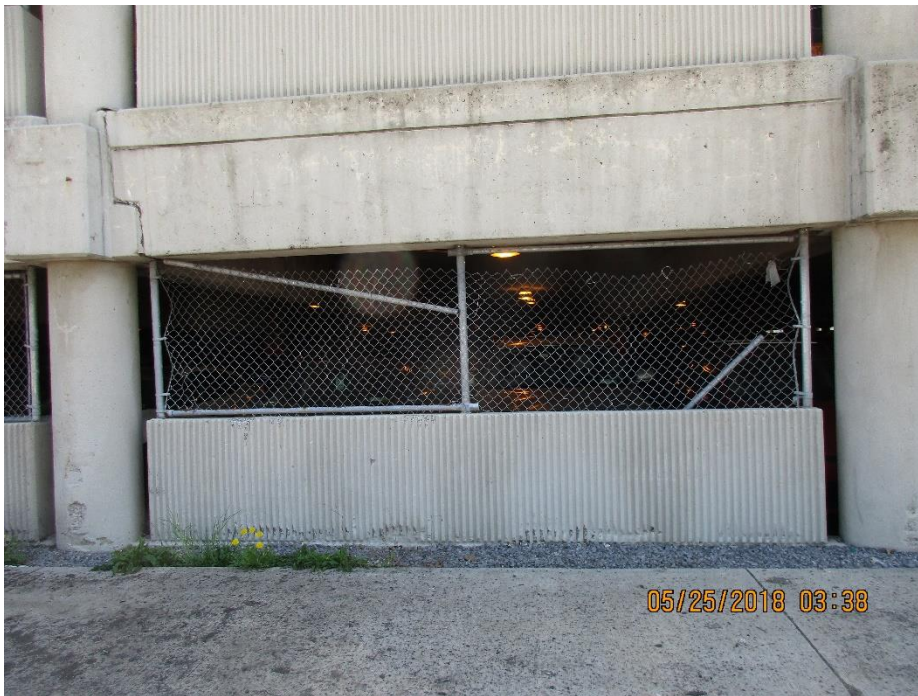
Photo #21: Damaged chain link fence on north side.
