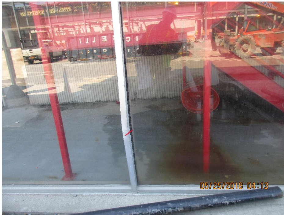
Photo #19: Damaged mullion at stair #1. Edge unsupported at glass panel.
