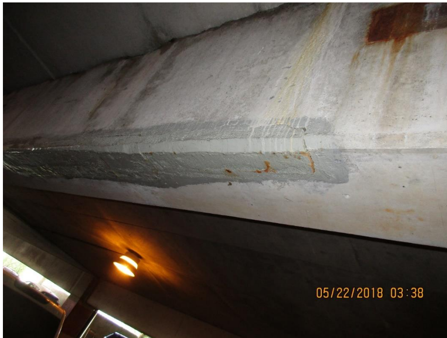
Photo #8: Level 3 Soffit-water leaking along the damaged joint at base of the South Ramp at the roof level. Also, crack along the patched area of girder.
