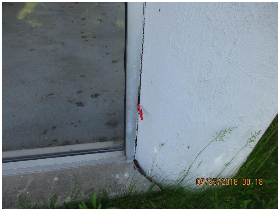
Photo #18: Failed caulk at Level 1 stair tower 3
