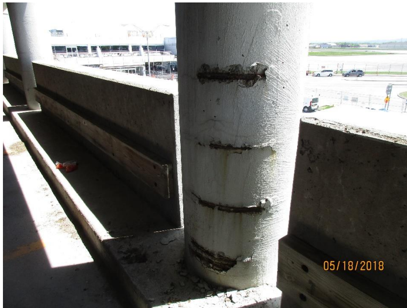
Photo #3: spalling concrete column with corroded ties on south end of Level 3
