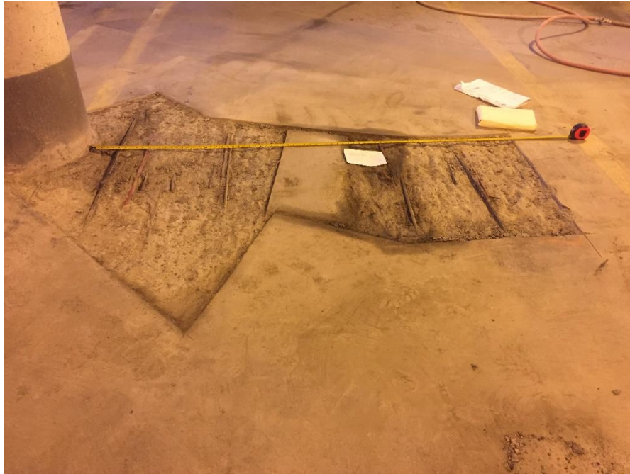
Photo #7: Two broken PTs at column C14 at Level 2.
