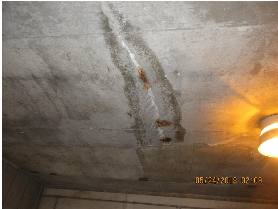
Photo #15: Level 2 soffit near column line Q30 – leaking crack with corrosion
