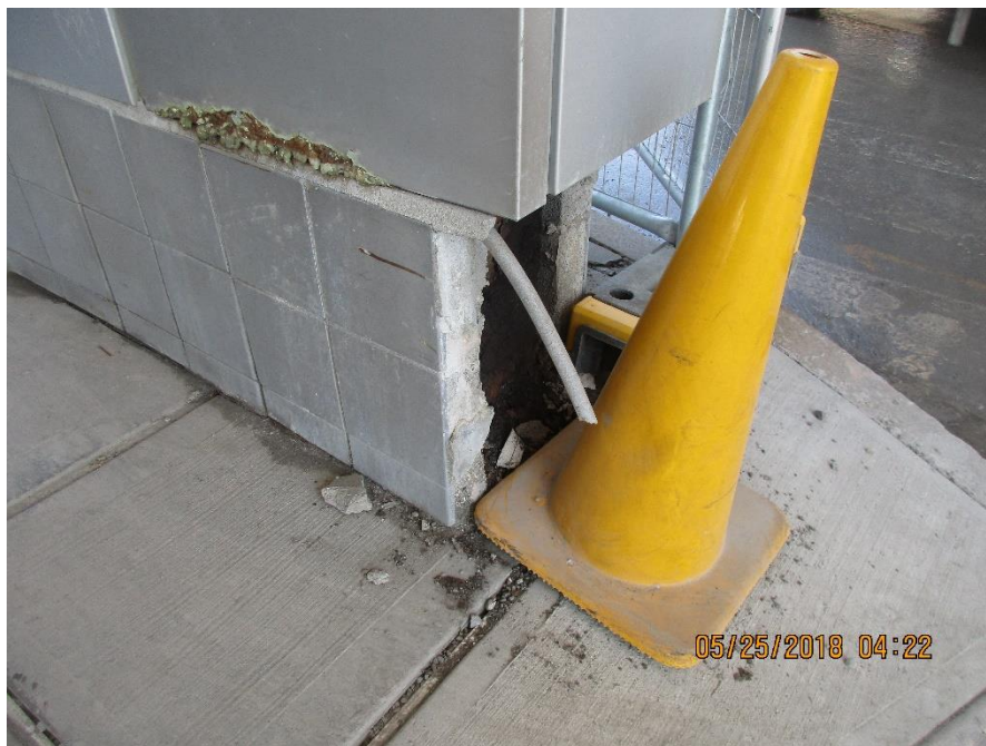
Photo #20: corroded steel column and damage glazed masonry at pedestrian bridge. We believe the glazed masonry was repaired.
