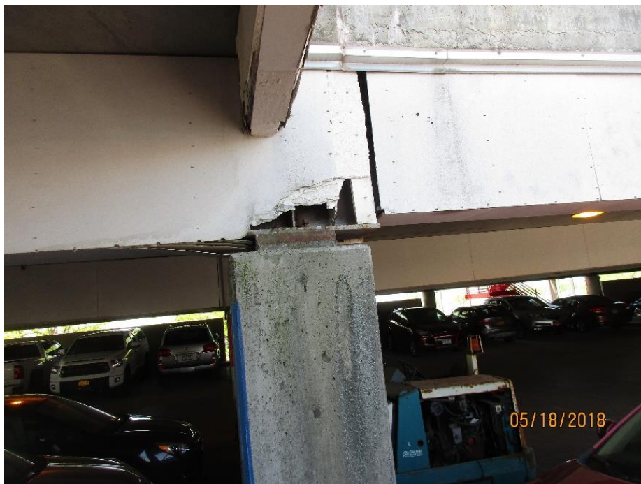
Photo # 10: Level 3- Roof Soffit- water damaged fireproofing board and corrosion of steel beam bearing plate.
