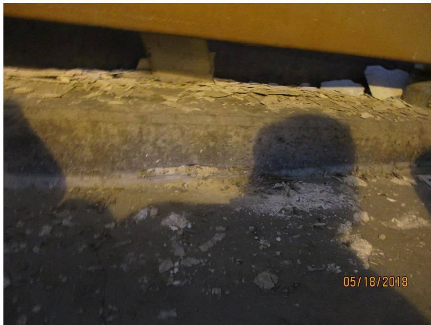
Photo #4: damaged fire proofing board falling on concrete deck near column line Q3 on Level 3
