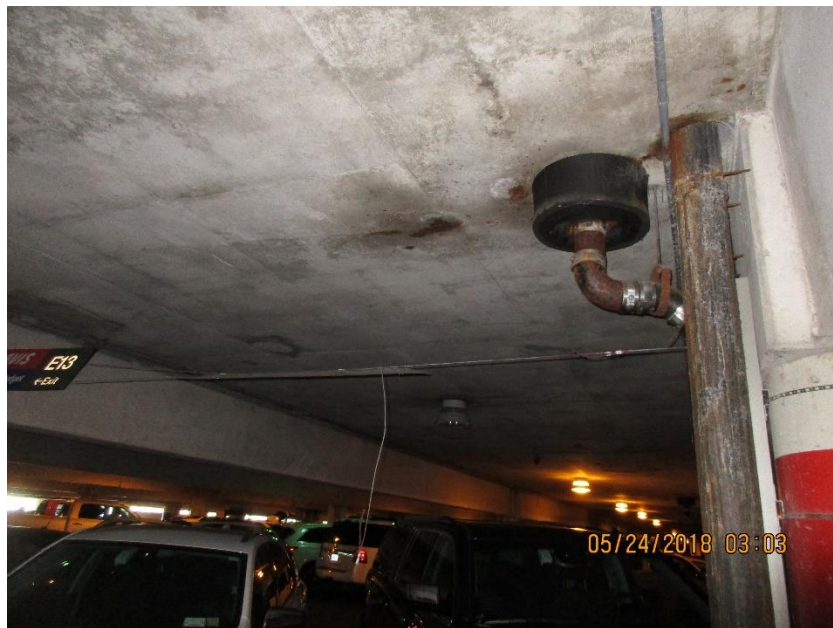
Photo #2: Level 2 Soffit-water stained concrete and corrosion at bottom of concrete deck at the floor drain. Typical condition below second floor. Broken rental car sign cable.
