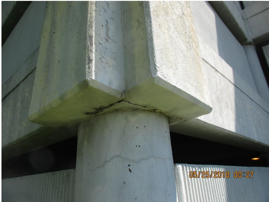
Photo #17: Cracked post tensioning pocket cover
