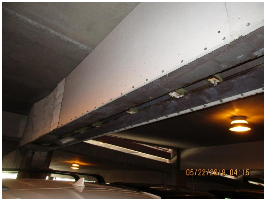
Photo #12: Missing fireproofing board at bottom of steel beam
