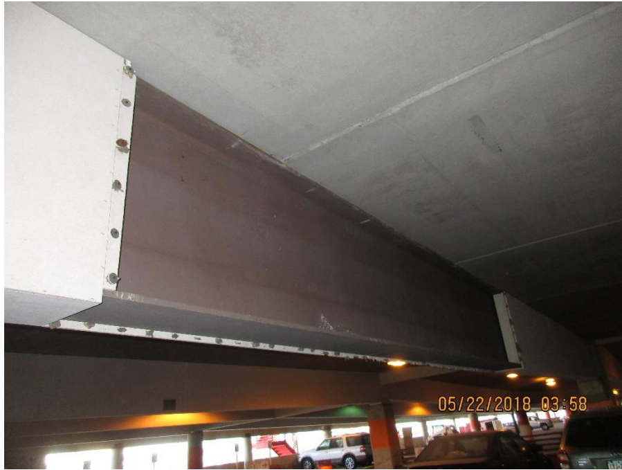
Photo #11: Level 3-Roof Soffit- missing fireproofing board at steel girder.
