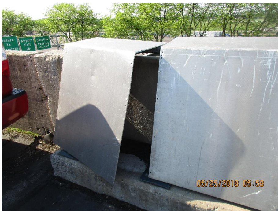
Photo #22: Loose section of snow deflector
