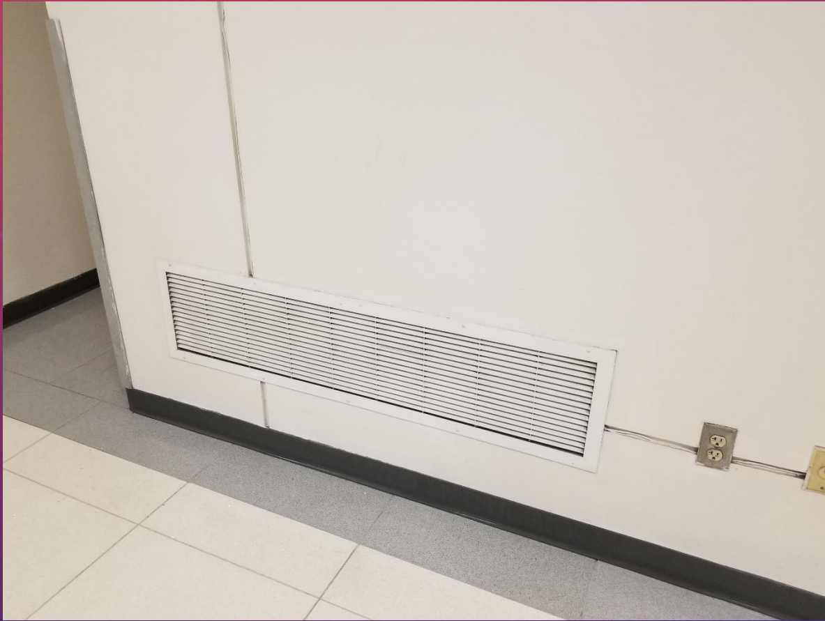
North Concourse - HVAC
